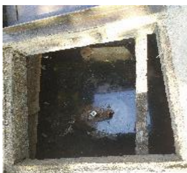
Near Karelibaug Overhead Tank Char Rasta (18 inches)
