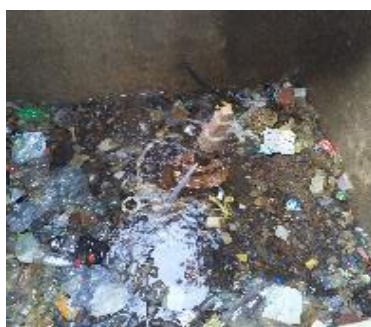
Opposite Indrapuri Pumping Station (18 inches)
